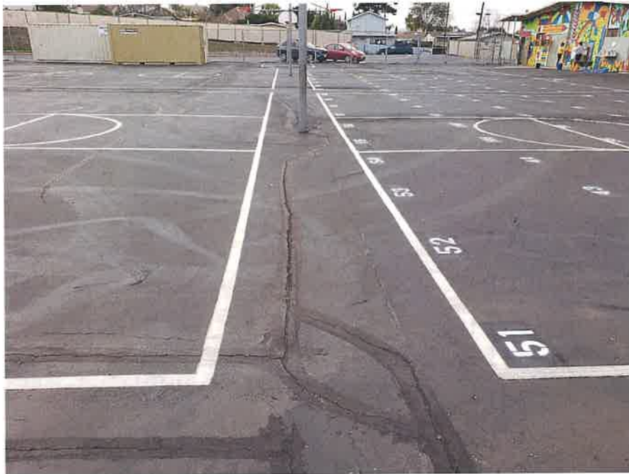
Photograph 7: West Hardcourt: View of play area looking west. Open cracks and previously patched cracks.
