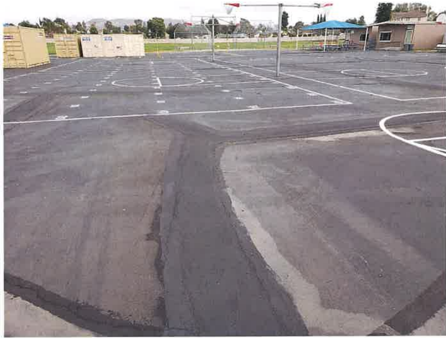
Photograph 5: West Hardcourt: Overall view of play area looking east. Open cracks and previously patched cracks.
