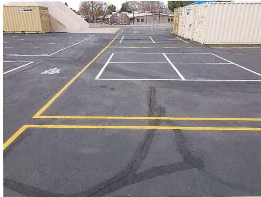
Photograph 6: West Hardcourt: View of play area looking north. Open cracks and previously patched cracks.
