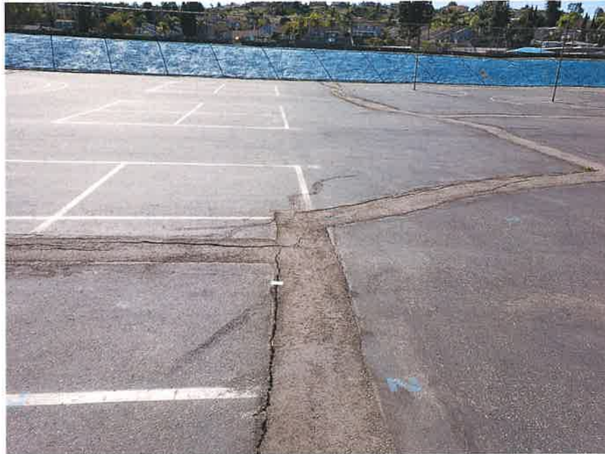
Photograph 3: North Hardcourt: View of play area looking south. Previously patched cracks reopening.
