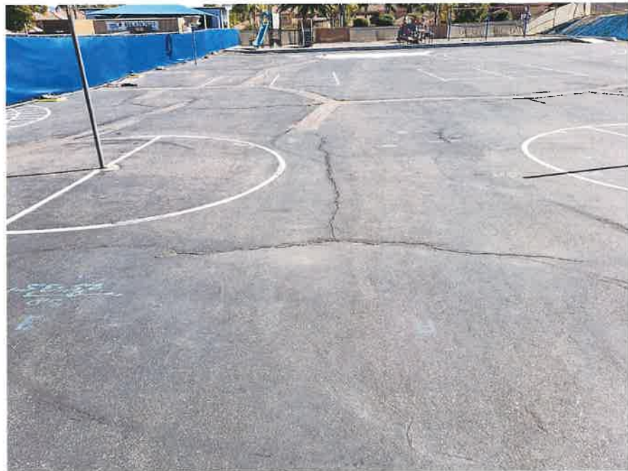
Photograph 2: North Hardcourt: View of play area looking east. Open cracks and previously patched cracks.
