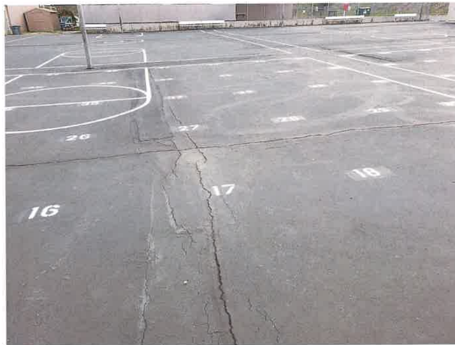
Photograph 8: West Hardcourt: View of play area looking south. Open cracks and previously patched cracks reopening.
